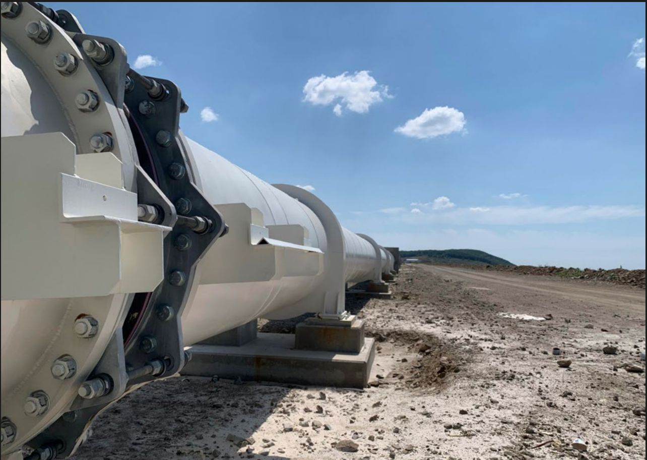
Installation of tied rubber expansion joints \varnothing 1,400 mm in a ring water line of a copper mine
