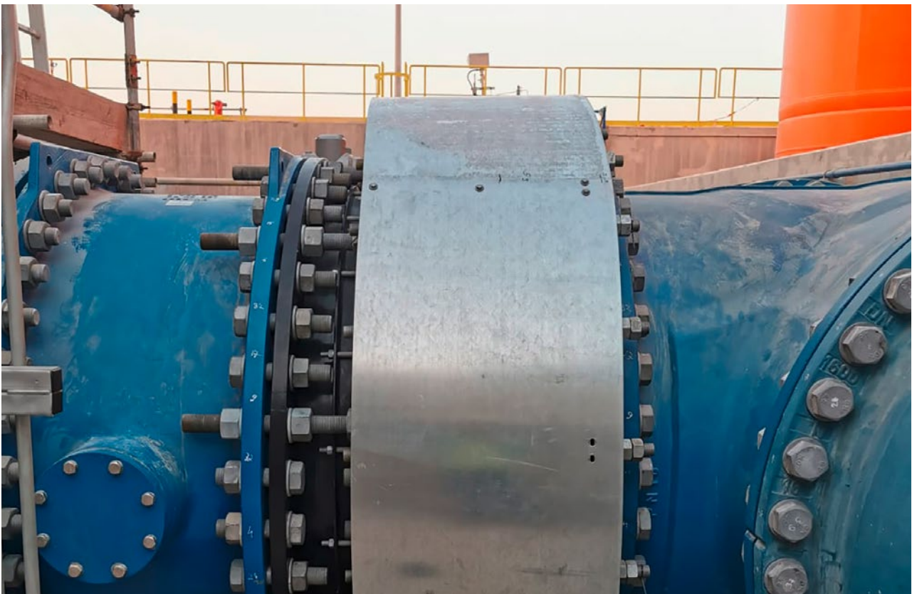
Metal protective cover against solar radiation
