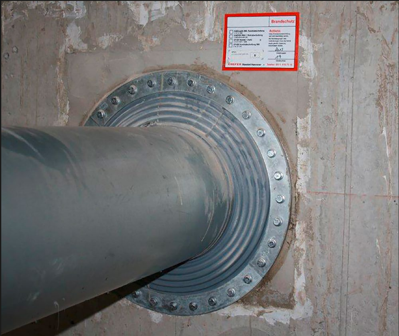
Fire protection bulkhead of type W200FS + W410FS for large pipe movements between machines house and boiler house
