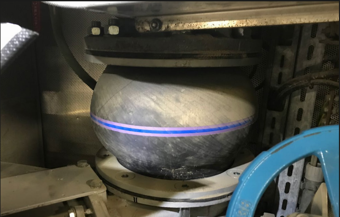
FPM rubber joint \varnothing 300 mm for 1 bar operating pressure and 180° C, installed on an ash chute
