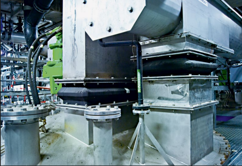
Elastomer expansion joints, type GU110 in the chute between the screw conveyor and sludge container in a slurry incineration facility ∅ 400 x 400 mm, 60 °C
