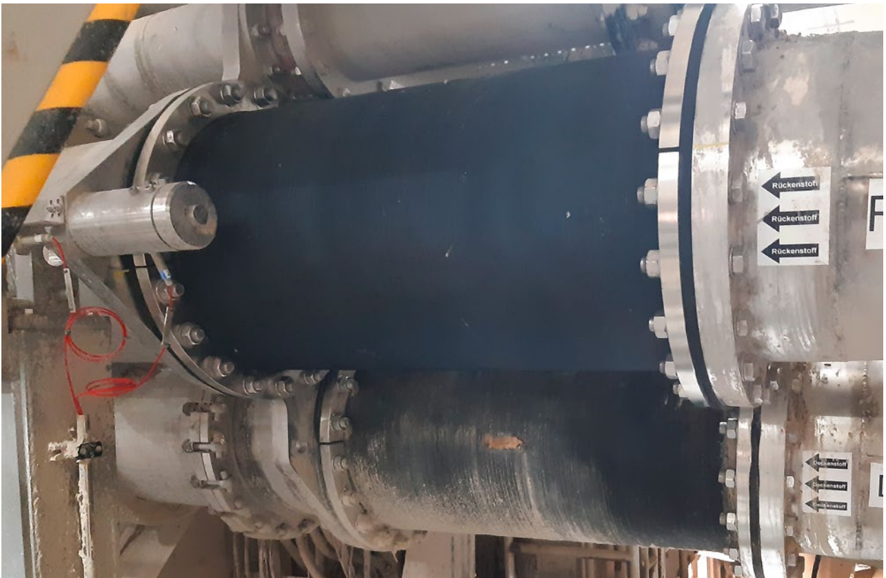
Replaced rubber flanged pipe in operation of a paper mill
