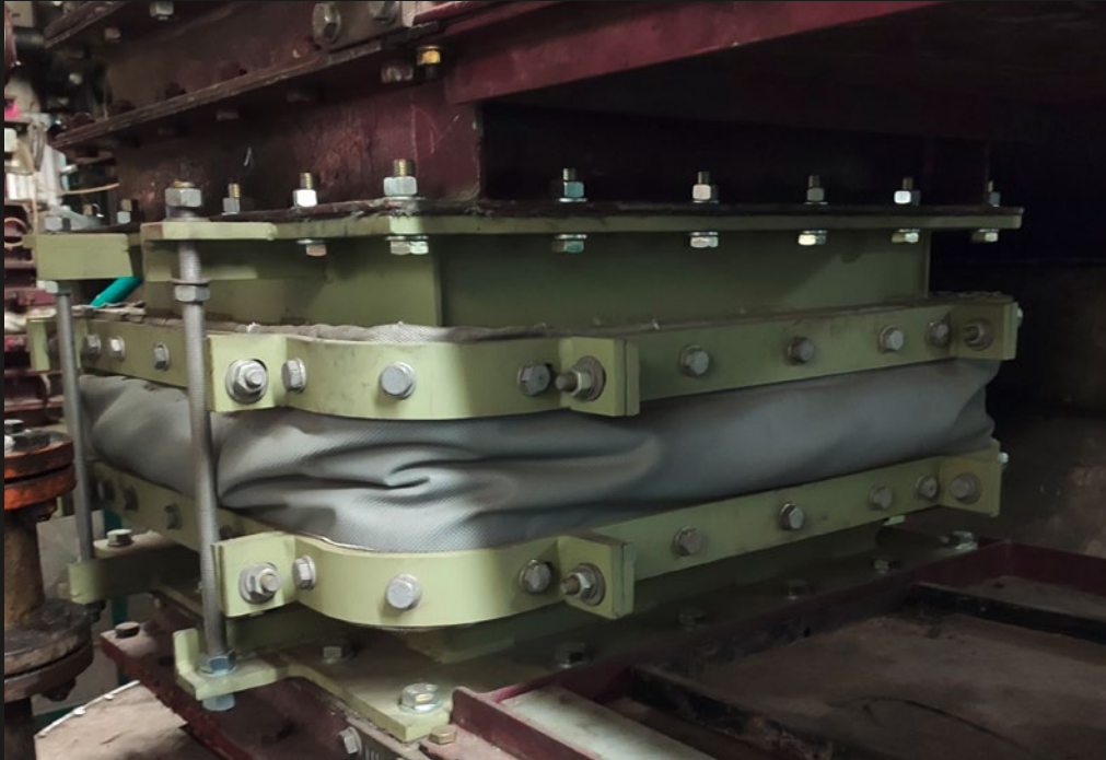
New fabric expansion joint installation unit at the ash outlet of a power plant
