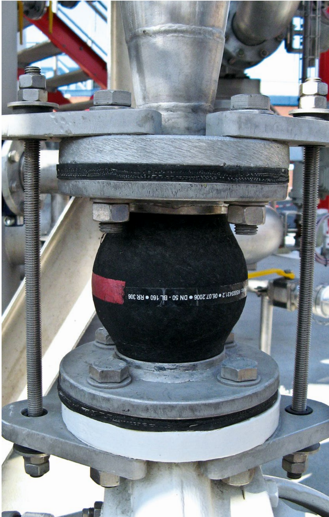
Lateral expansion joint, type U110R on the pump pressure side in a paper mill Ø 50 mm, 10 bar
