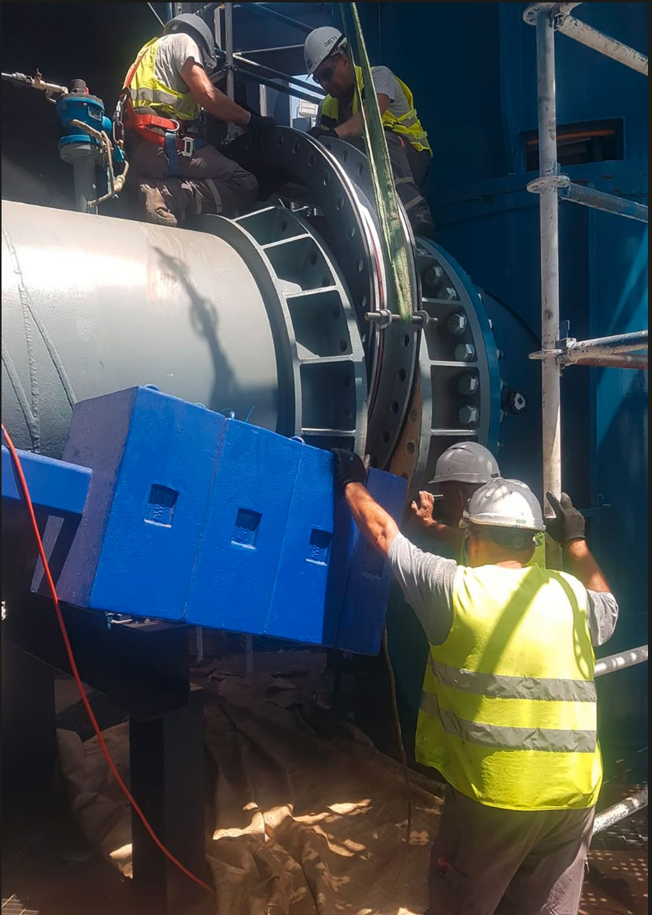
Installation of a rubber expansion joint \varnothing 1,600 mm to the pump nozzle, 16 bar design pressure
